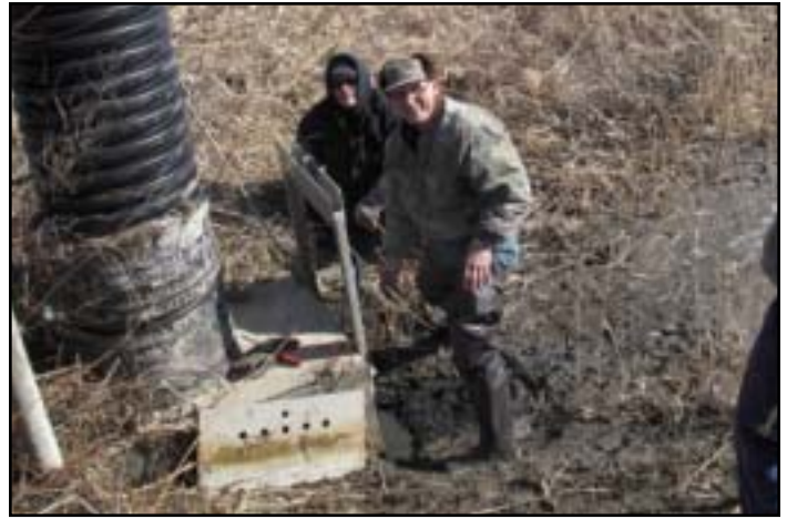
Ryan Terzaghi (left) and Richard Koch working on the drain pipe at the Walleye ponds on the Selfridge ANG Base earlier this spring."
